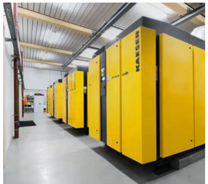
The four HBS rotary screw blowers from KAESER.
