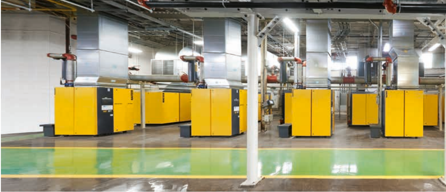
Image left: The new compressed air station is a technical and visual highlight. Image right: SIGMA CONTROL 2 efficiency centre.
