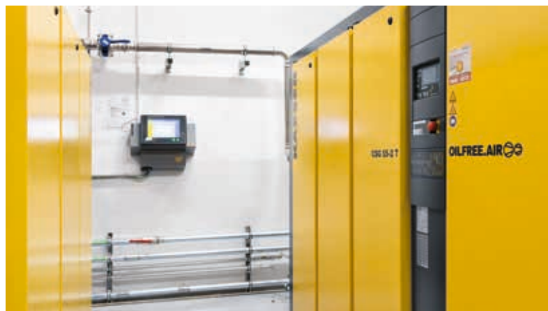
The SIGMA AIR MANAGER 4.0 ensures energy-efficient control at all times.
